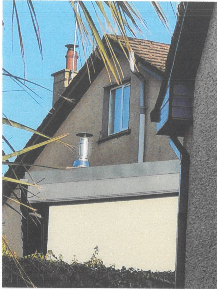
Picture 5: Showing gable window on the side elevation of attic (no planning application on file for this window) and chimney flue of extension.
