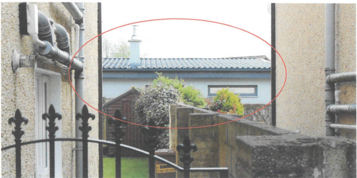
Picture 2: Picture taken from public path outside houses no 37, 38. Shows metal/aluminium clad roofing, not slates or tiles.
